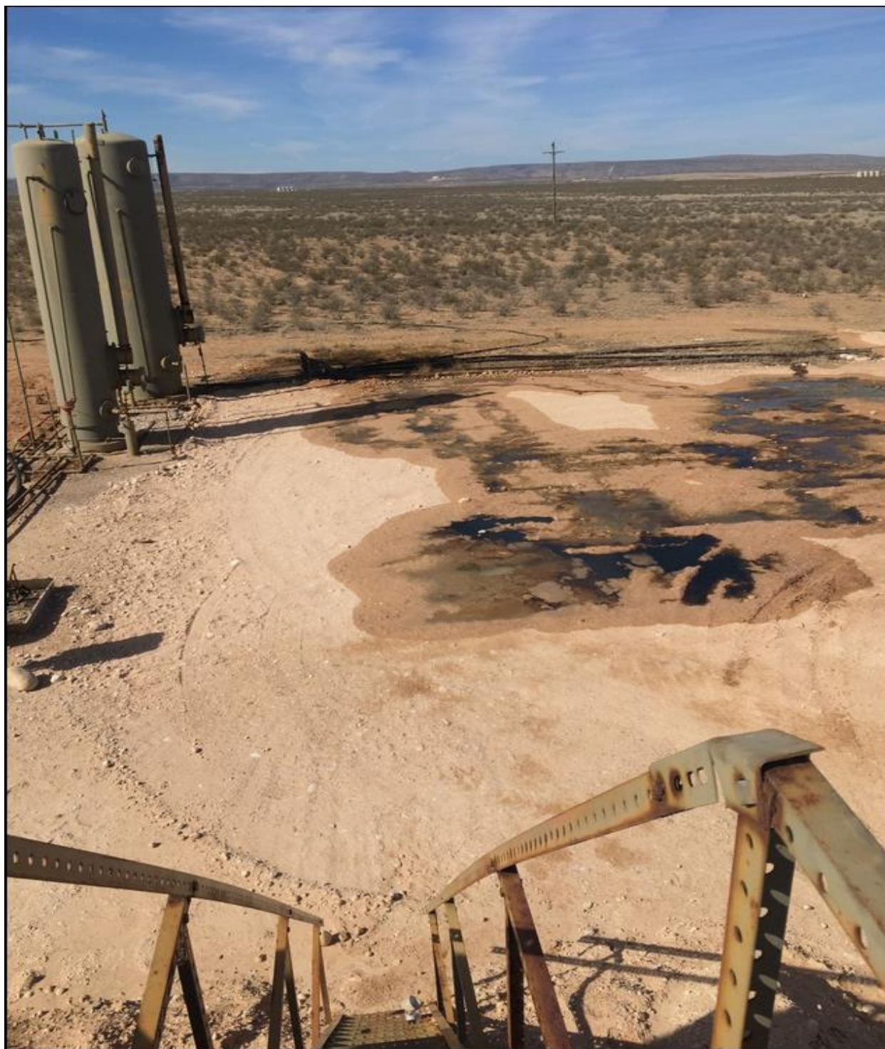
Bandit State #4 Tank Battery looking west.
