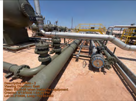
BS25-06 taken underneath the equipment
