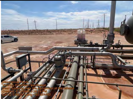
Looking over the equipment at the southwest area of the release
