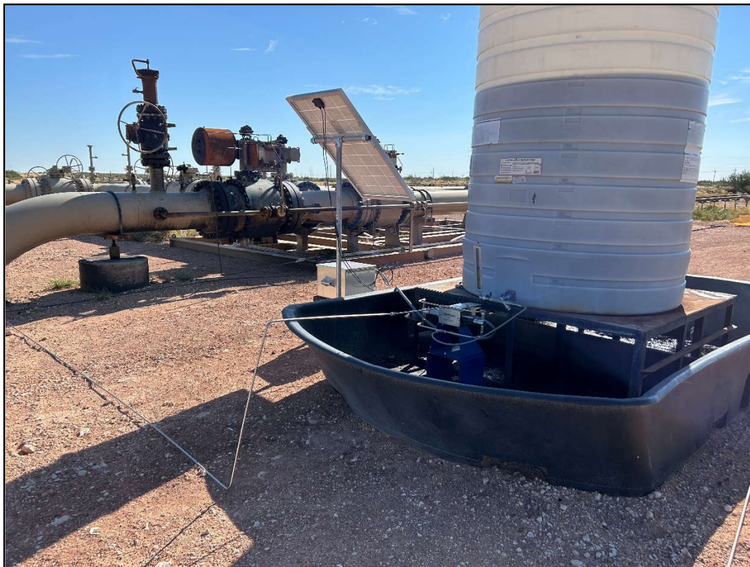
Photo of Chemical Tank and Auto Launcher facing south
