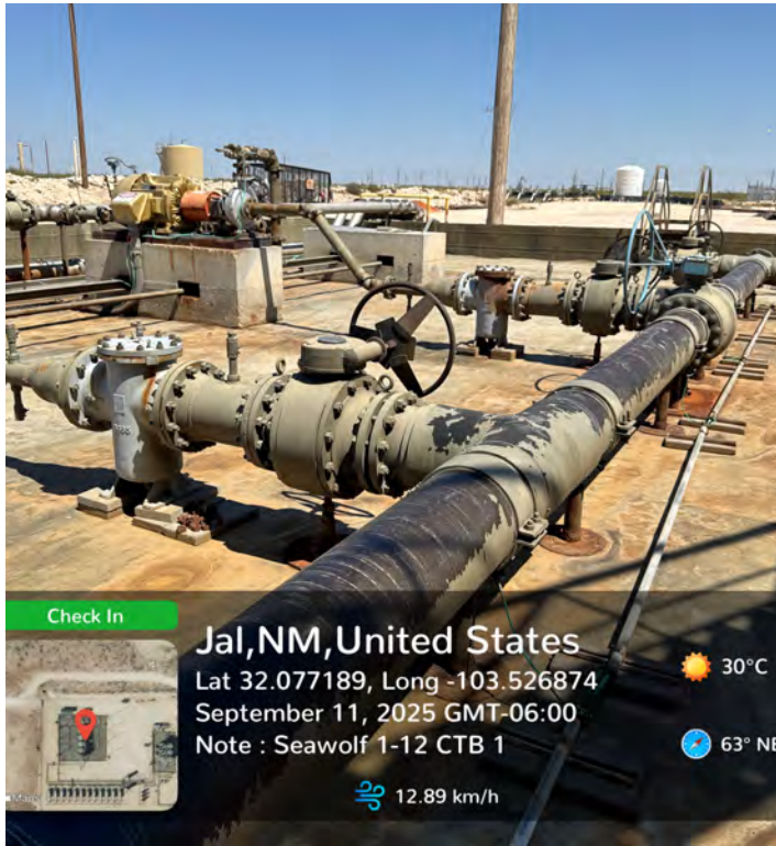
Northeast corner area near pumps and piping.
