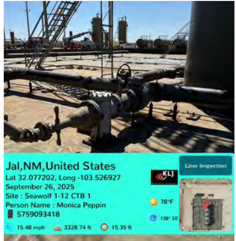
North area near pumps and tanks facing west.
