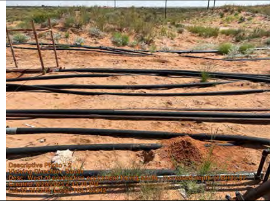
West of production equipment facing south.
