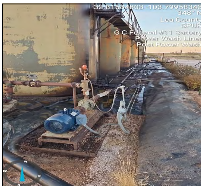
Photo of location taken post power wash facing north.
