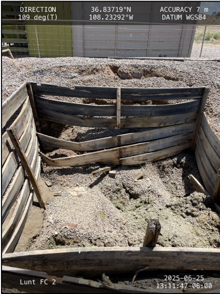
Photograph: 1 Date: 06/25/2025 Description: Release Area within below-grade tank pit View: Southeast
