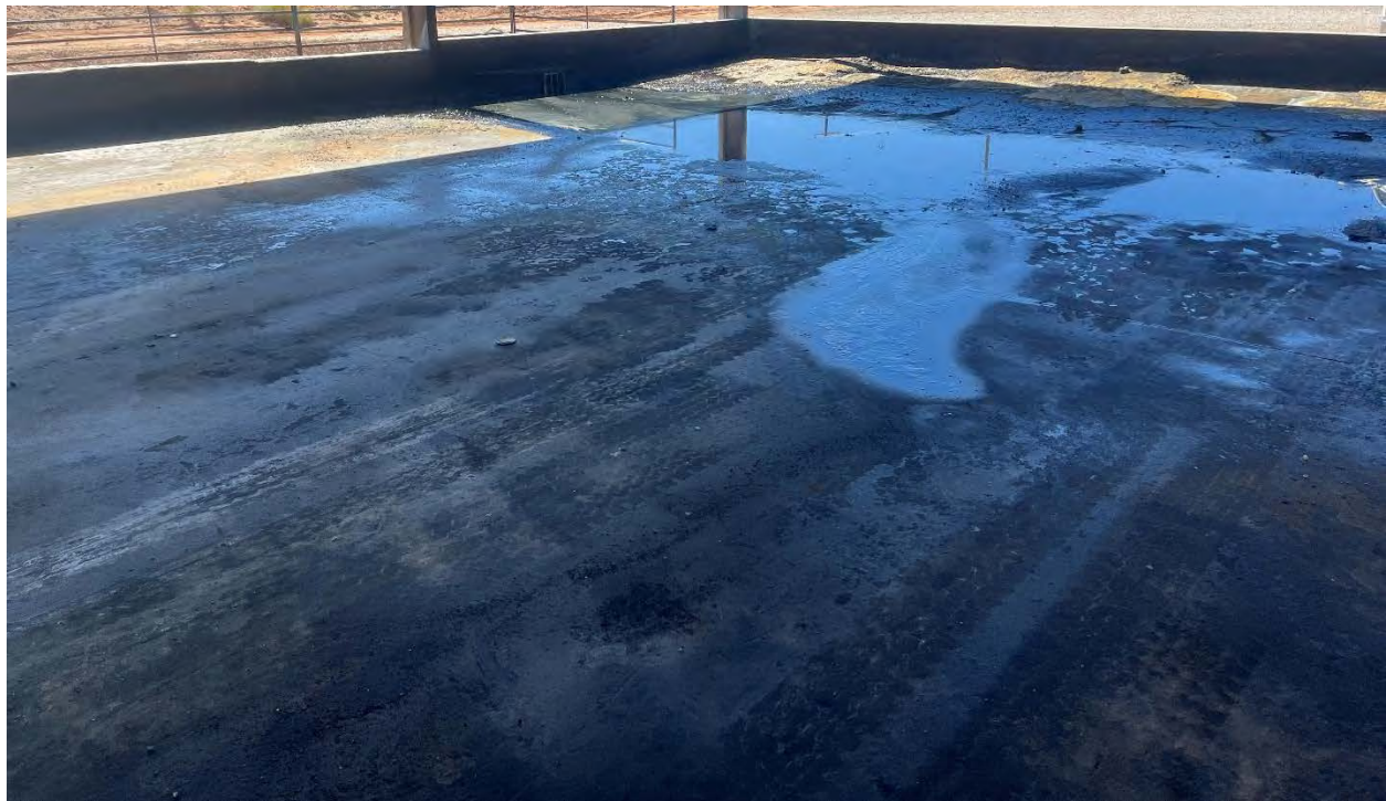
Image 8. Center of Washout pad showing sloped drain area
