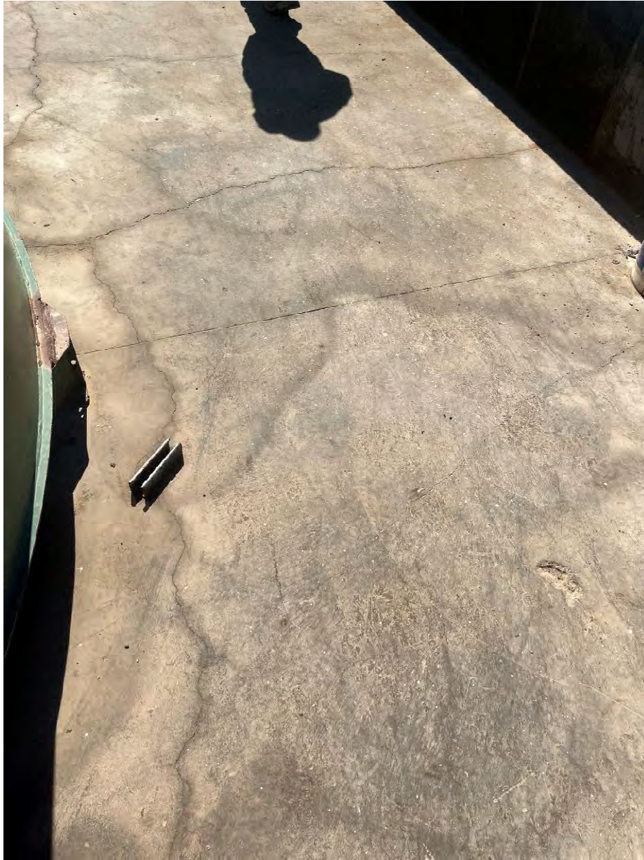
Image 5. Shrinkage cracks between tanks of the secondary containment
