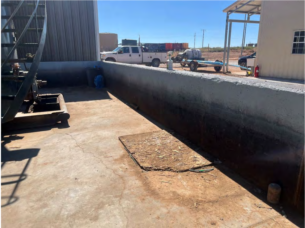
Image 6. Discoloration of the inside South Perimeter Wall
