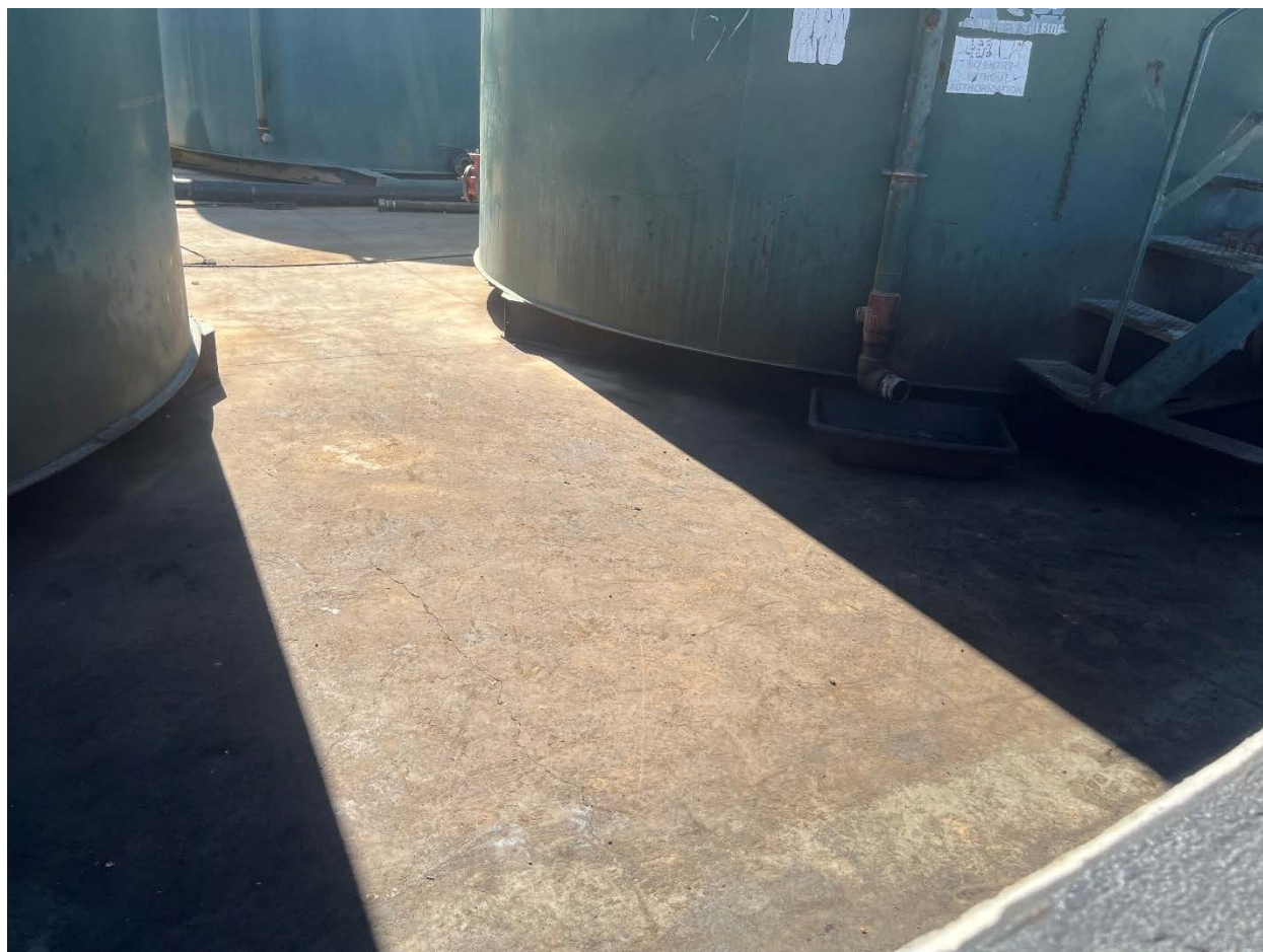
Image 1. Random shrinkage cracks between tanks of the secondary containment
