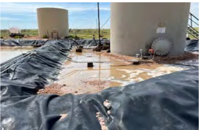
View to S of Battery containment (9/17/25).
