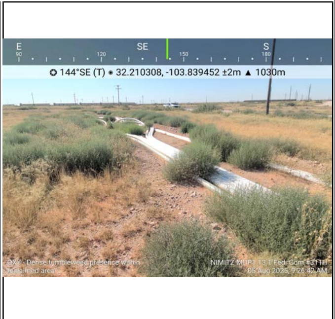
Photograph 2 Date: 08/05/2025 Description: Utility lines and undesirable tumbleweed View: Southeast
