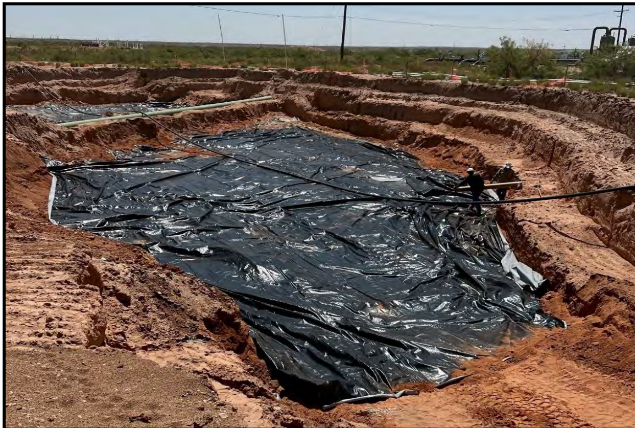
View of liner placed in excavation area prior to backfill, facing southeast.
