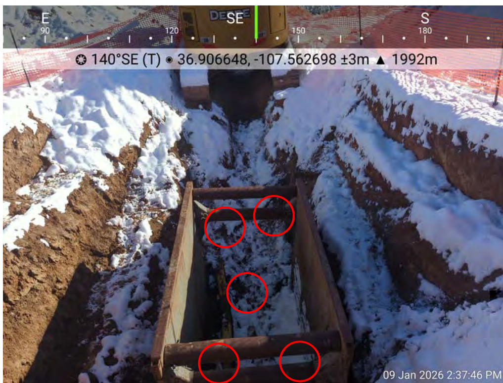
Photo 13: SS11 is a five-point composite sample collected from base of excavation area.
