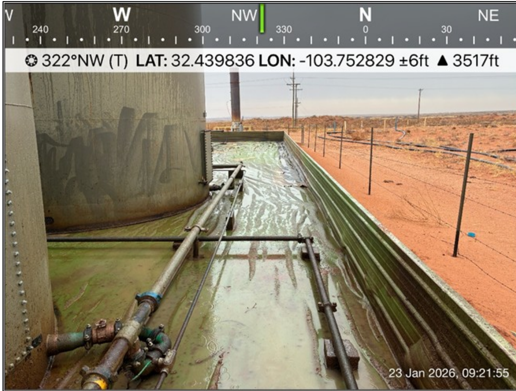
PHOTO 5: Northwestern view following initial pressure washing activities and weather events. 1/23/2026
