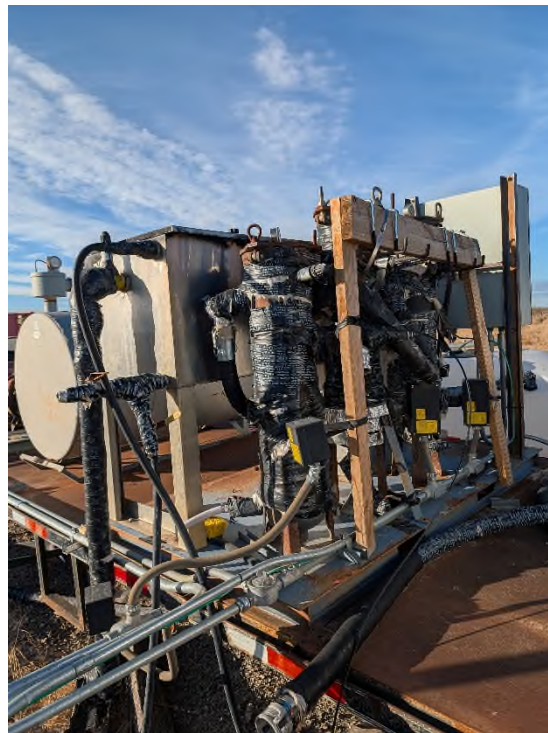
Photograph 6 Pump and Treat recovery system on a trailer.
