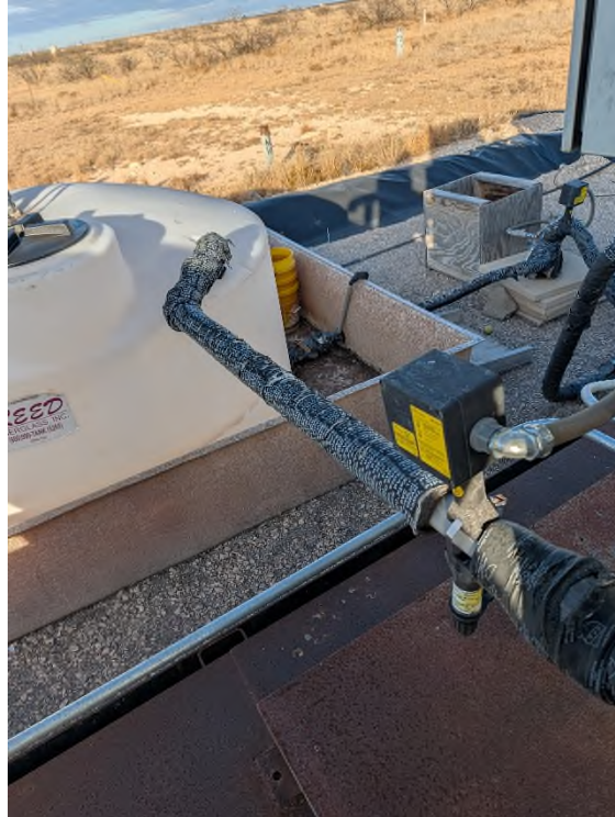
Photograph 5 Another view of the Air sparging tank in a containment pan that is part of the Pump and Treat recovery system in poly line containment.
