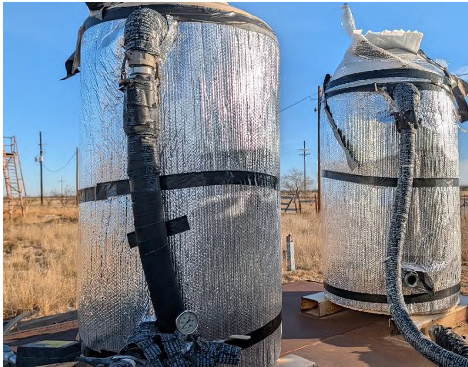
Photograph 8 Carbon vessels that are part of the trailer mounted Pump and Treat system.
