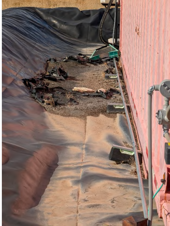
Photograph 3 Frac tank within poly line containment.
