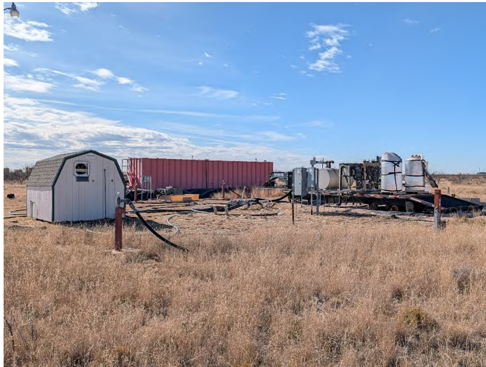
Photograph 2 Shed with compressor, Frac tank with and Pump and Treat recovery system in poly line containment.
