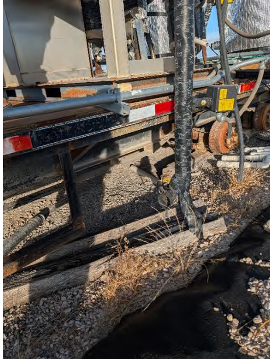
Photograph 7 Containment berm around trailer mounted Pump and Treat system.
