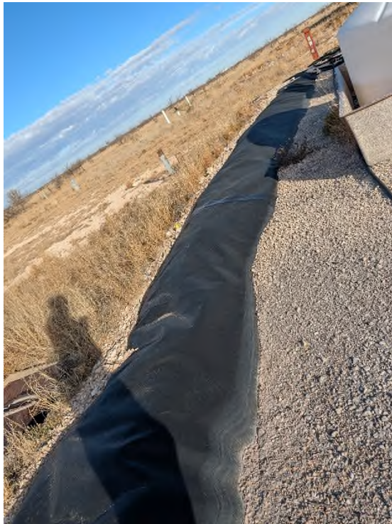
Photograph 4 Air sparging tank in a containment pan that is part of the Pump and Treat recovery system in poly line containment.
