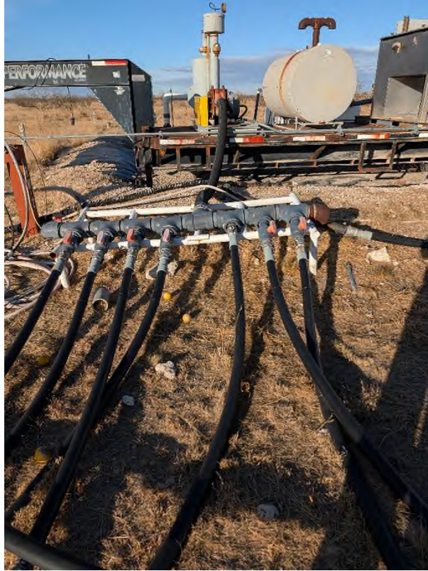
Photograph 9 Air line connections from the blower to the air sparging wells, trac tank and air sparging tank.
