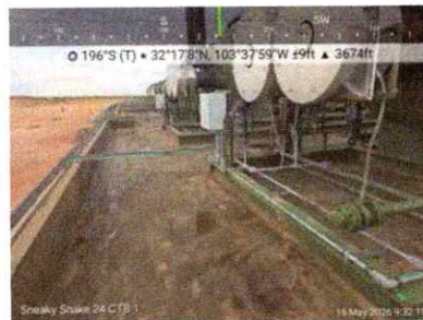
#45 Secondary containment — south berm edge, compressor skid
