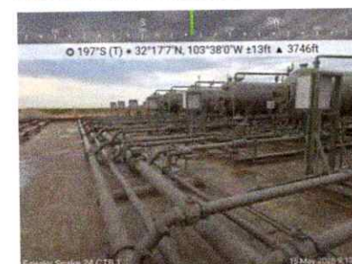
Secondary containment — manifold berm, south view 09:13:51 197°S 32°17'7"N 103°38'0"W
