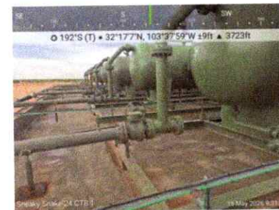
#42 Secondary containment — south view, separator vessel row 09:31:34 192°S 32°17'7"N 103°37'59"W
