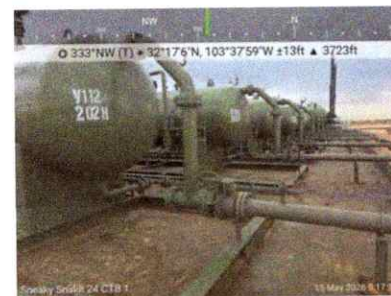
#41 Secondary containment — NW view, V112/202H and V110/302H 09:17:36 333°NW 32°17'6"N 103°37'59"W
