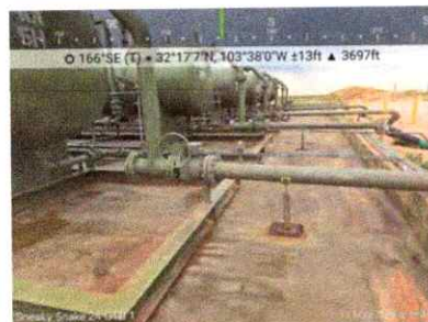
Secondary containment — berm surface, separator vessel row 08:38:46 166°SE 32°17'7"N 103°38'0"W
