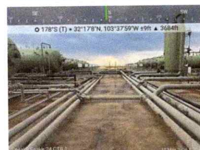
Secondary containment — manifold area, south view
