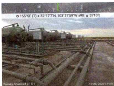
Secondary containment — separator vessel row, SE view, V-104/4H 09:14:05 155°SE 32°17'7"N 103°37'59"W
