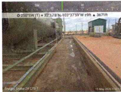
#44 Secondary containment — west berm edge, SW view
