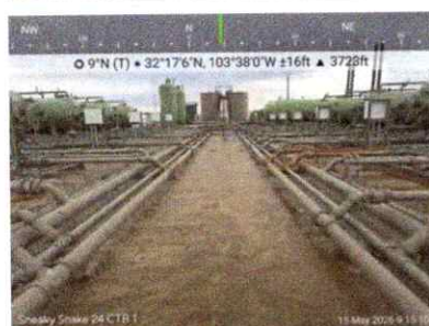
#39 Secondary containment — manifold berm center, north view 09:15:10 9°N 32°17'6"N 103°38'0"W
