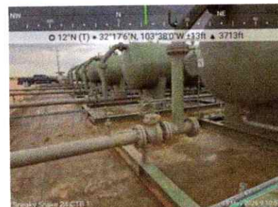
Secondary containment — north view, V117/302N 09:10:57 12°N 32°17'6"N 103°38'0"W
