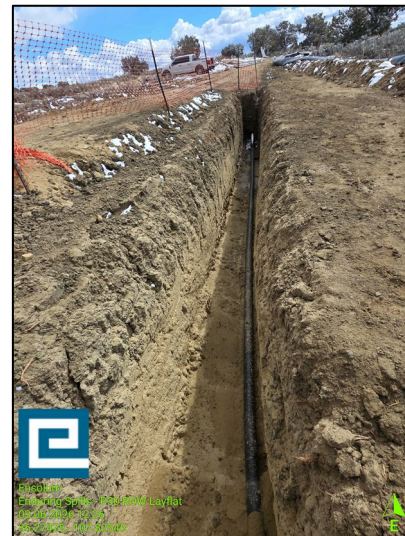
Photograph: 4 Date: 3/6/2026 Description: Pipeline trench and sampling areas SS07 through SS09 View: North
