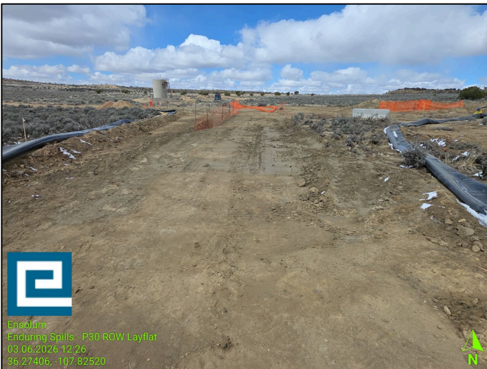
Photograph: 3 Date: 3/6/2026 Description: Initial sampling activities to assess soil conditions, sampling areas SS01 through SS06 View: North
