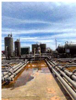
Photo 3 of 5 - Spill Across Pipeline Skid
