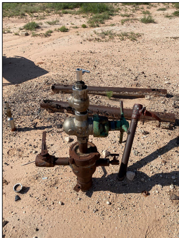
3) Twin Lakes SA #086 (30-005-60794) – Wellhead
