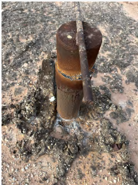
CSA #196: South Wellhead
