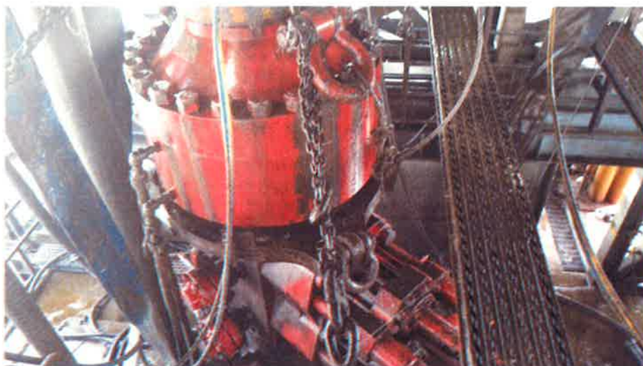
Figure 1: Winch System attached to BOP Stack
