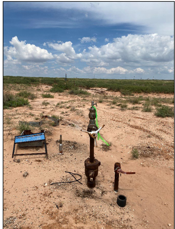
4) TLSA #78K (30-005-60995) – Methane Monitoring Complete
