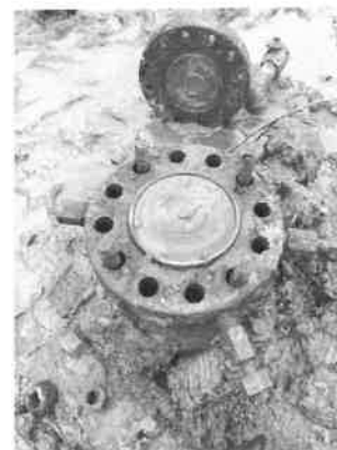
Cement standing at surface
