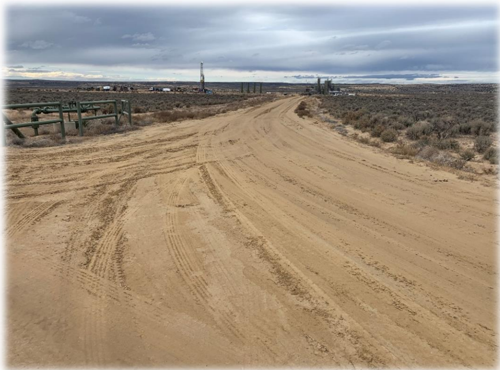
Photo 5. Existing Access Road and Well-Connect Pipeline Start Looking North terminating at existing well pad.
