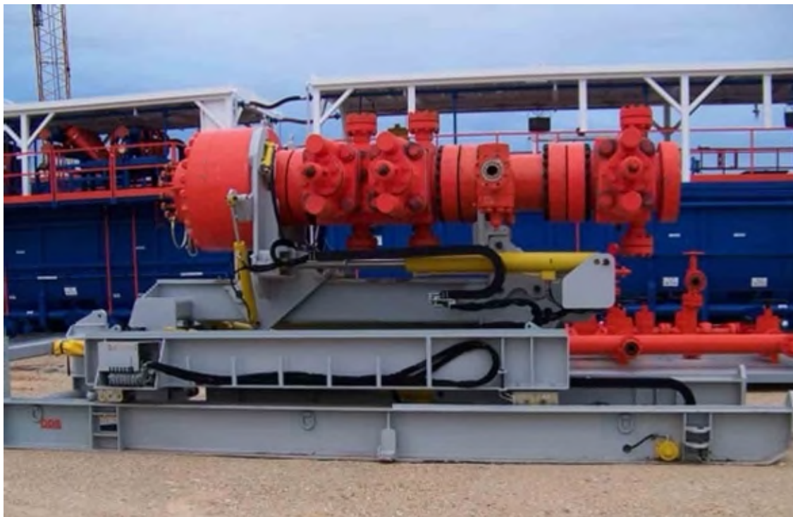
Figure 4. BOP handling system
