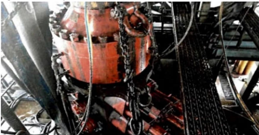
Figure 1: Winch System attached to BOP Stack
