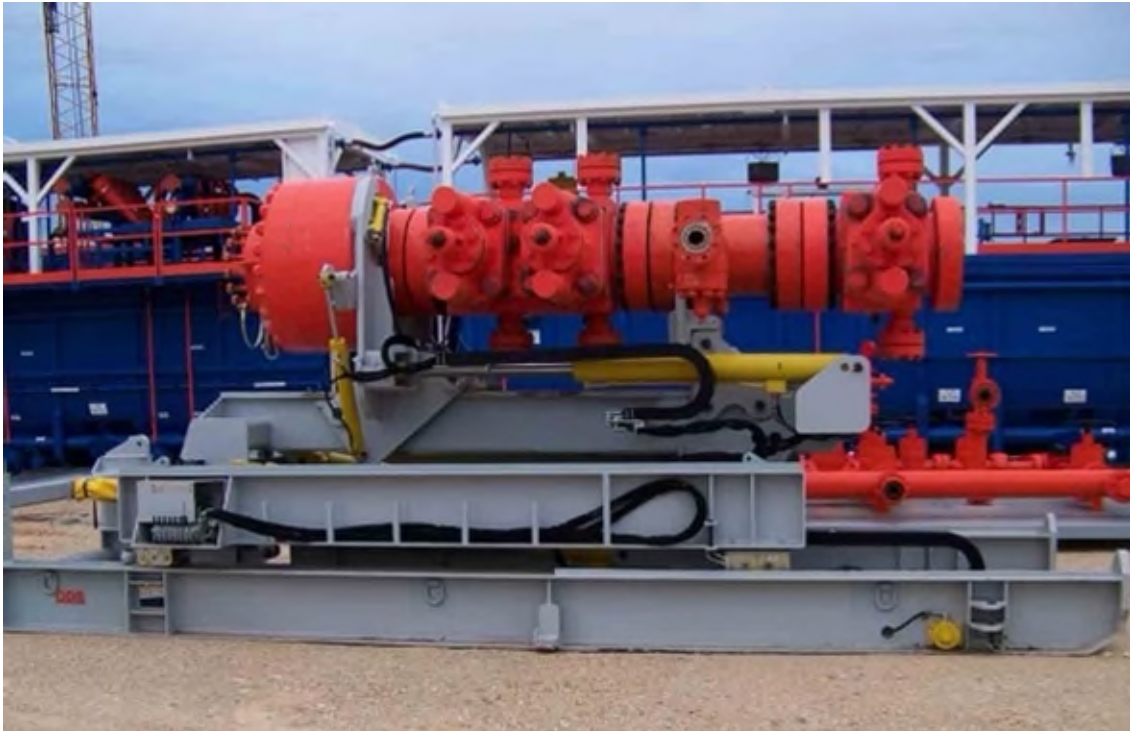
Figure 4. BOP handling system
