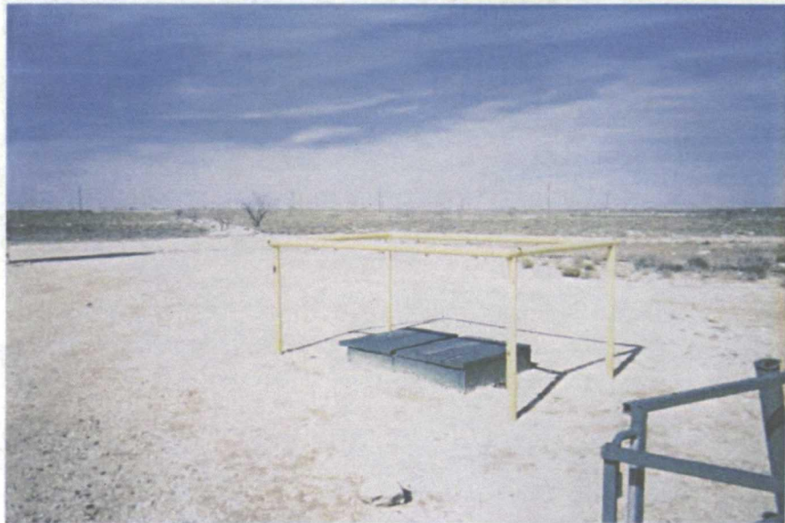
undisturbed junction box (1)
