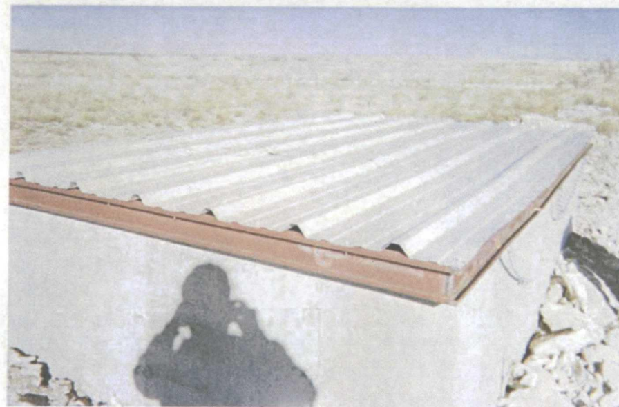
new, watertight junction box
