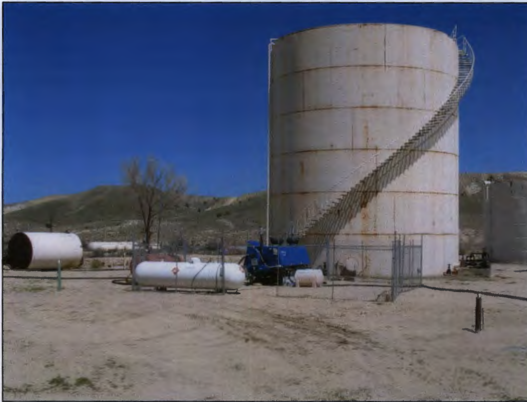
1. High vacuum extraction system located on south side of tank #18
