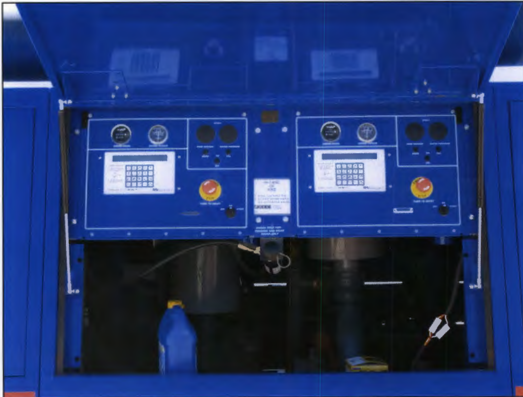
3. RSI system control panels
