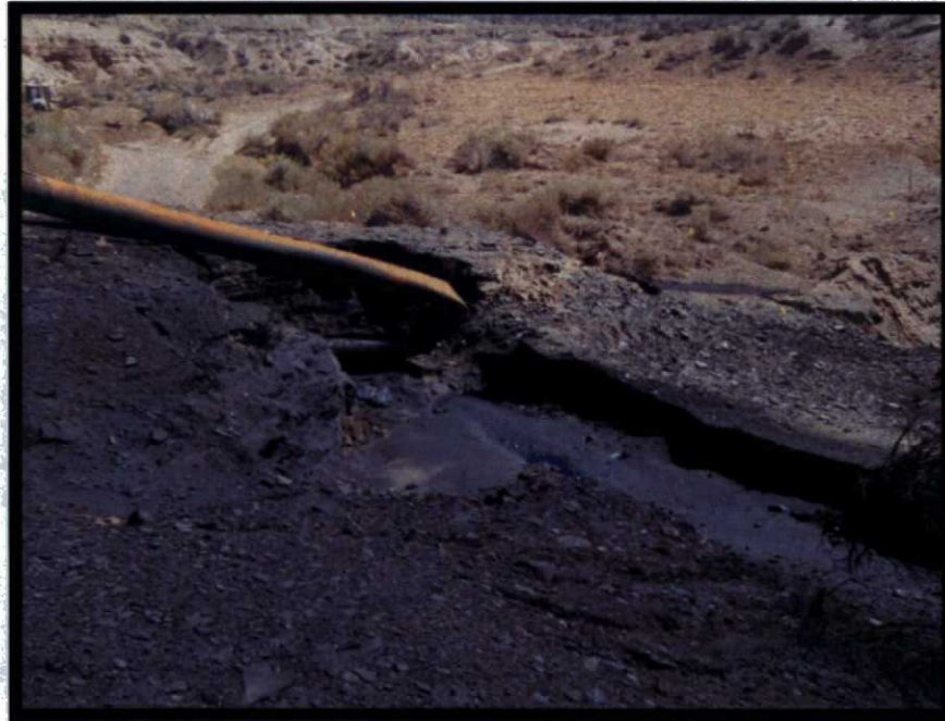
Photo 1: Initial Response View 1
