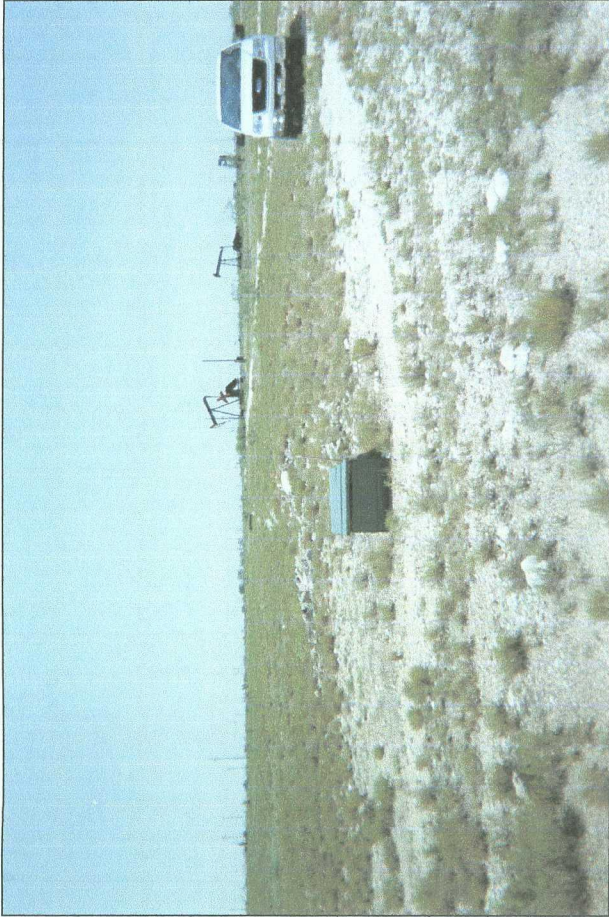
undisturbed junction box
