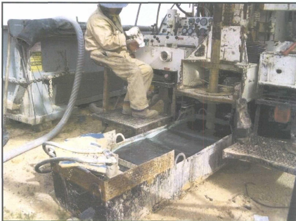
Cuttings separator box with oil, April 2009
