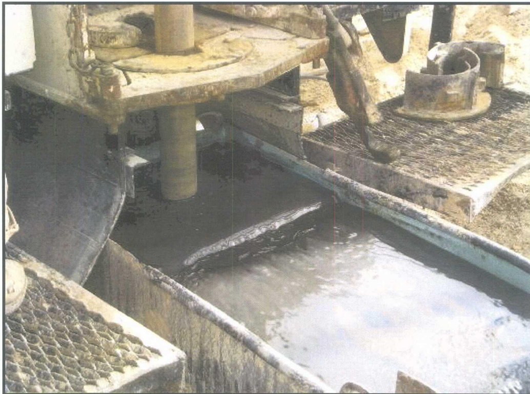
Cuttings separator box with oil and hydrocarbon sheen, April 2009
