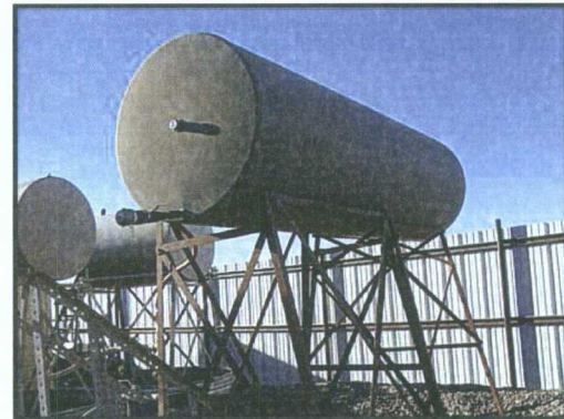
Photo 9: Insure all tanks are labeled
