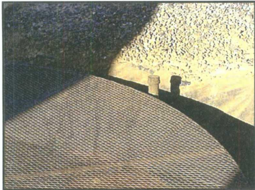
Photo 6: Tank is double bottomed. The spout pictured is to check for liquids/leaks between the bottoms.
