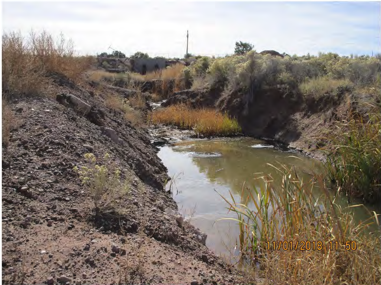
Photo No. 2: Looking south along retention ditch, midway between north and south ends. Some hydrocarbon staining along perimeter of ditch, but very little hydrocarbon present on water. Location of concentrated hydrocarbon discharge at upper (southern) end of this ponded area.
