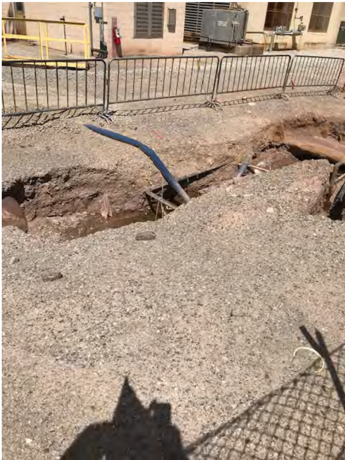
RO reject line (temporary) going to Pond 9.
