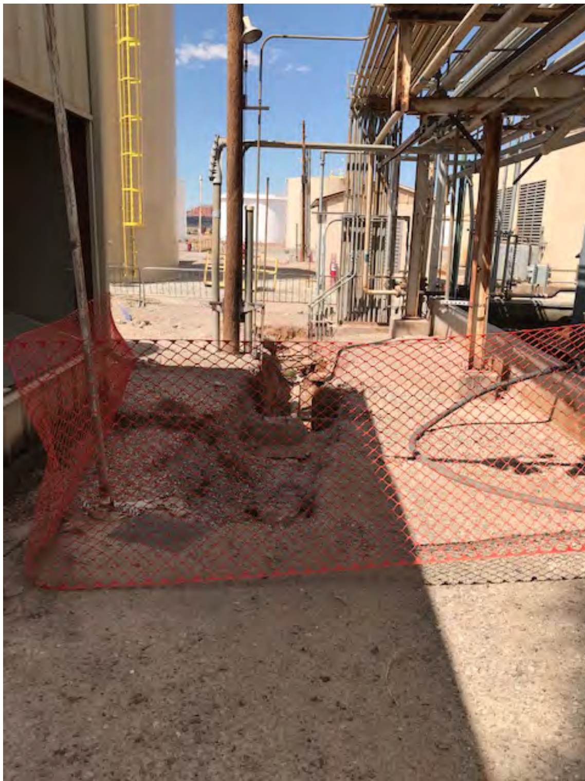
RO reject line coming from water treatment buildings near de-aeration unit.
