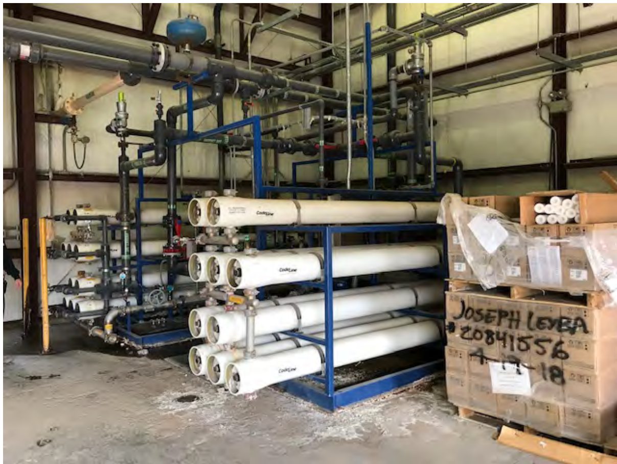
Step 2: Reverse Osmosis water softening system.
