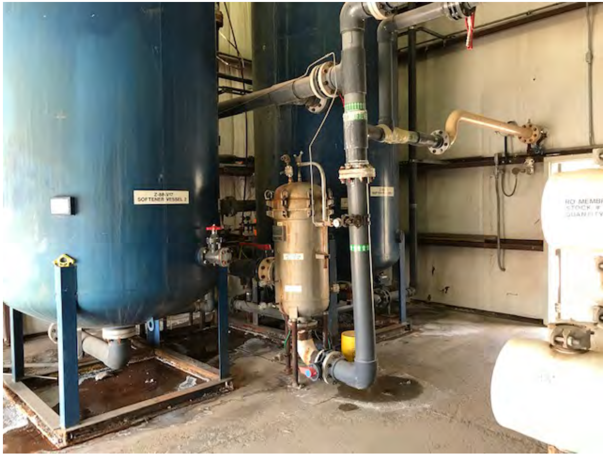
Step 1: Water softening unit.
