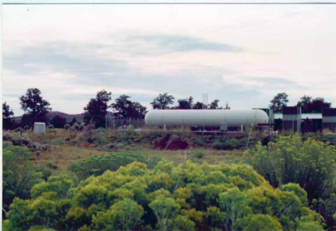
30,000 Gallon Tank & EPNG Sales
