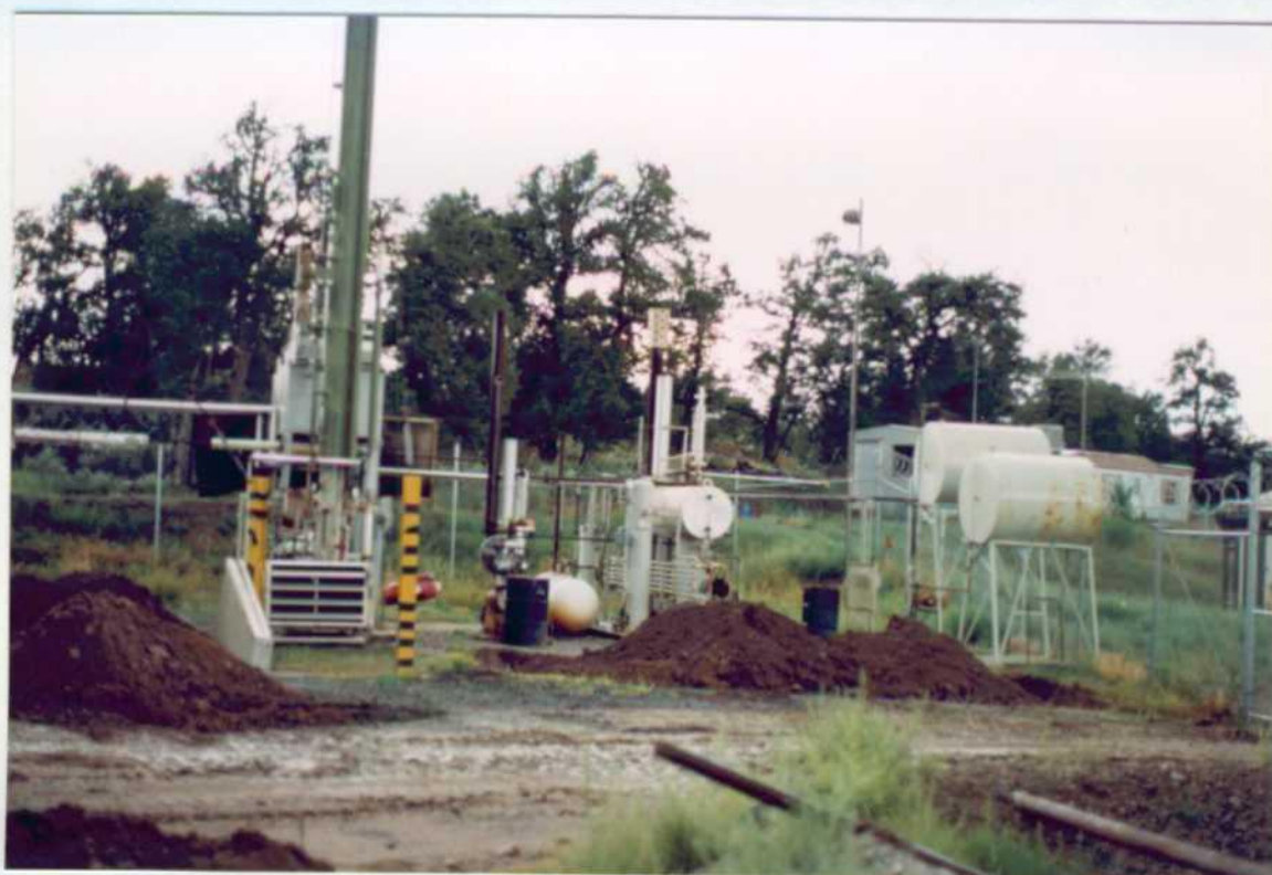
Heat Exchange Process Equipment
