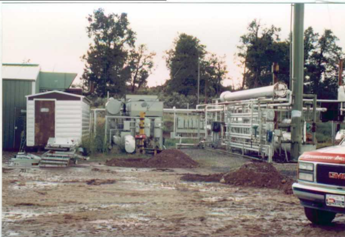
Heater / Treater Equipment
