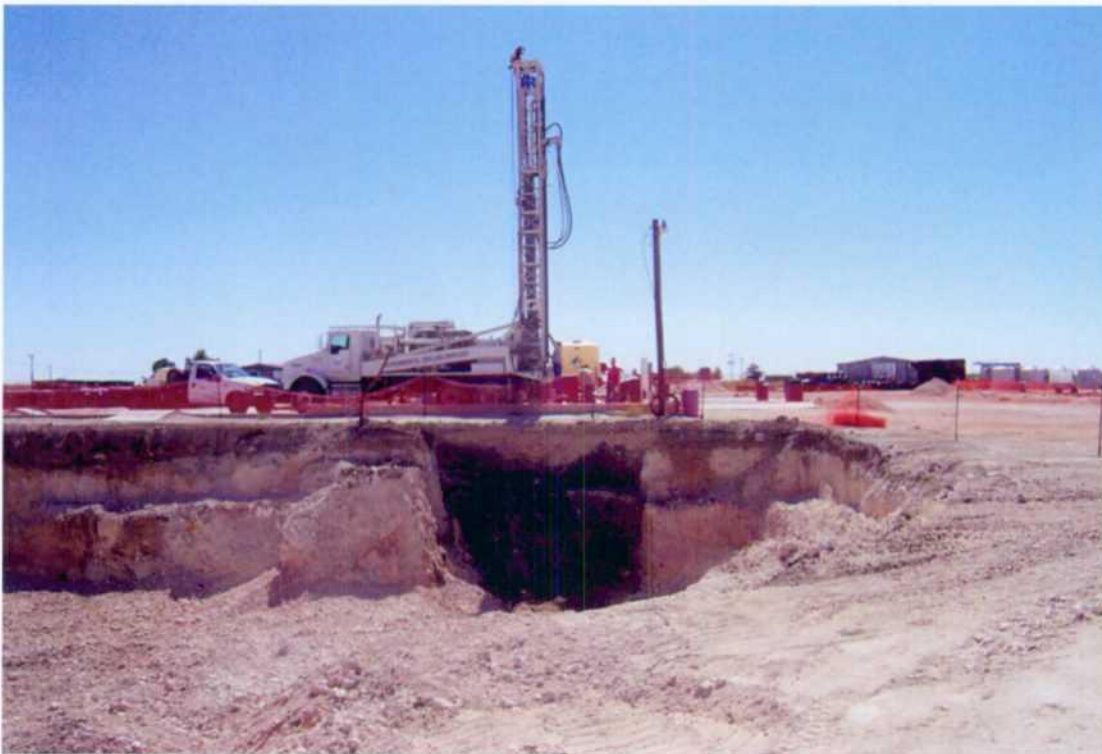
View south. Placement of soil boring SB-57 above stained south side wall (9-27-02).
