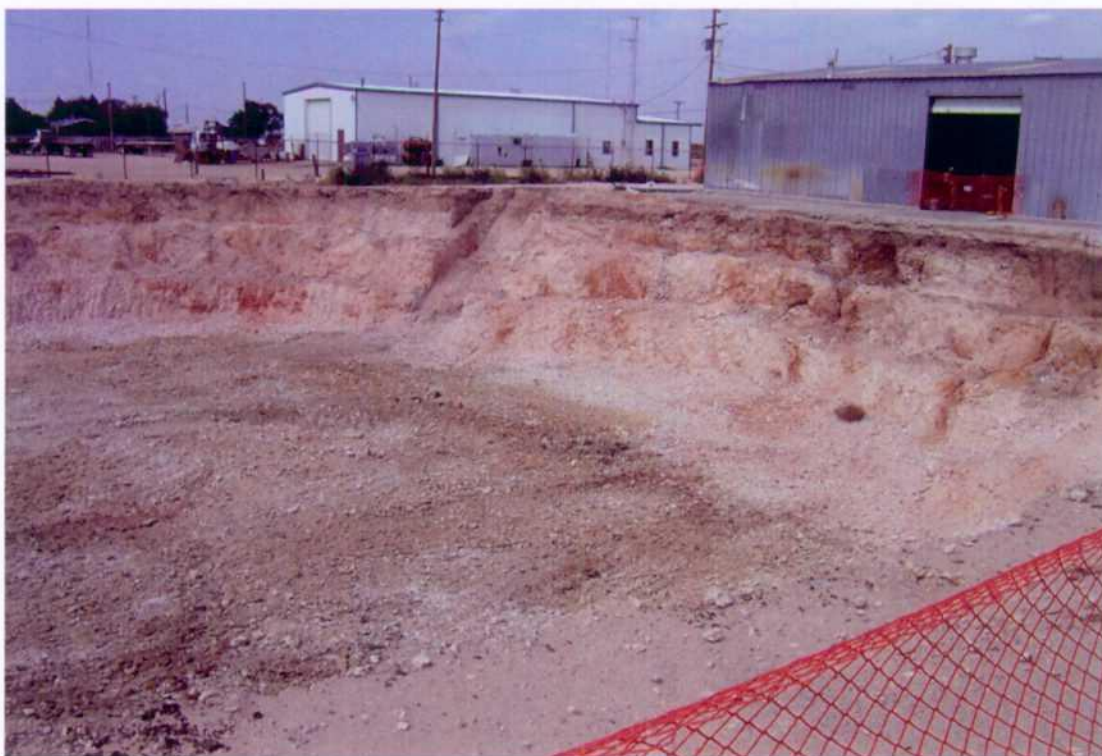
View north-northeast. North & east sidewalls, stain on bottom. (8-09-02).
