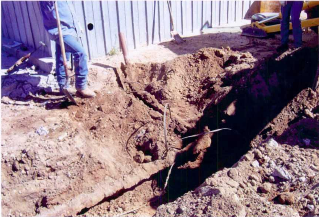
Drain system pipelines from warehouse (10-4-02).
