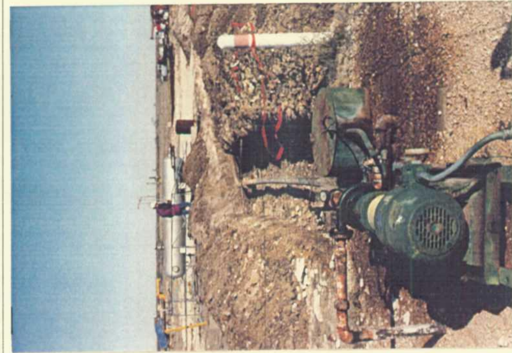
Photograph No. 9 Exposed Production Pipe Line looking north.
