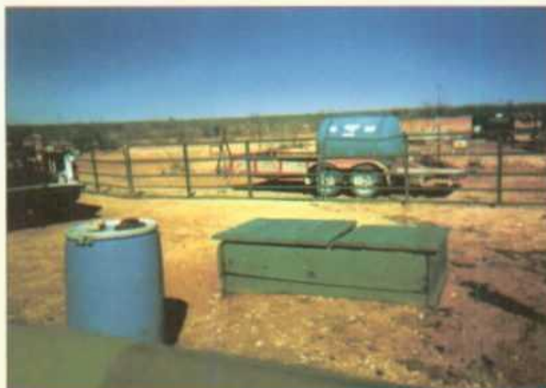
Old Junction Box
