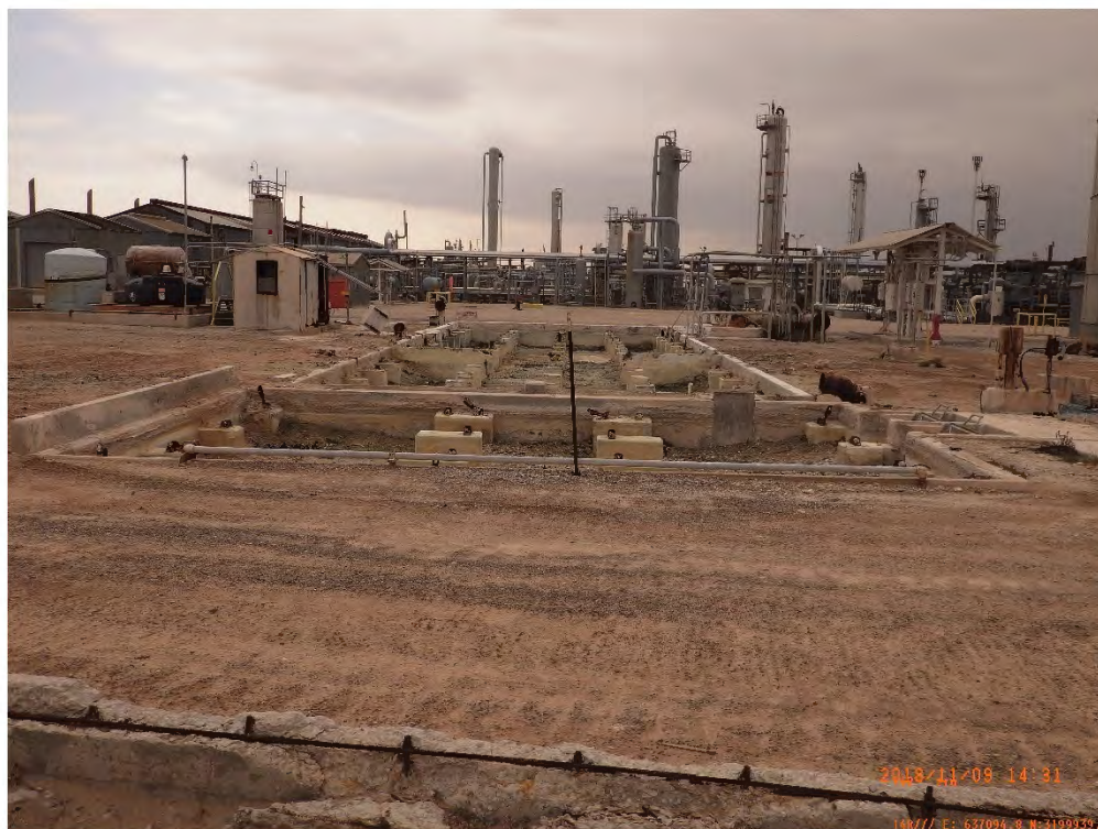
Cooling Tower Location Viewing South
