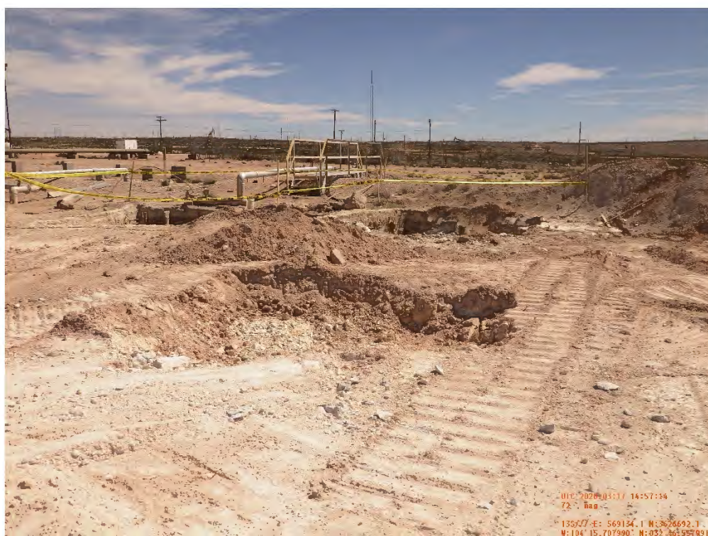
Slop Oil Tanks Location Viewing Northwest, March 25, 2020
