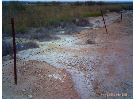
Salt Stain On Backside of Battery
