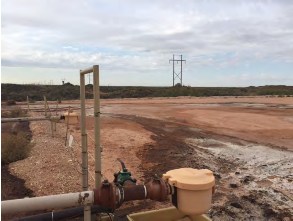
Lost Tank 33 Federal #2 SWD – Release (Looking Southwest)
