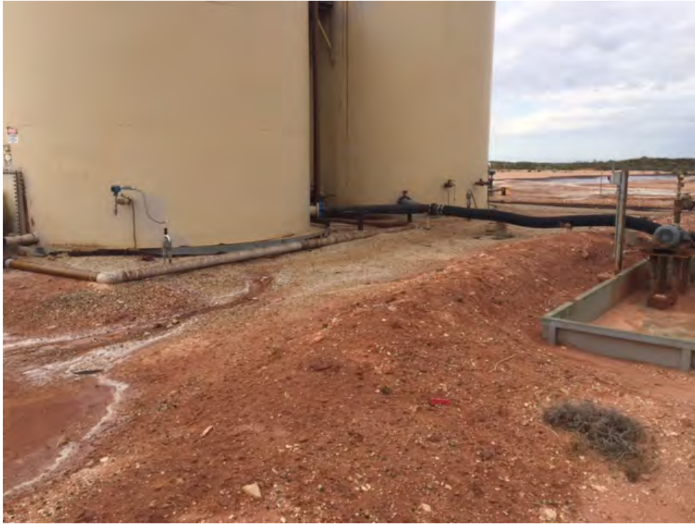
Lost Tank 33 Federal #2 SWD – Release (Looking West-Southwest)
