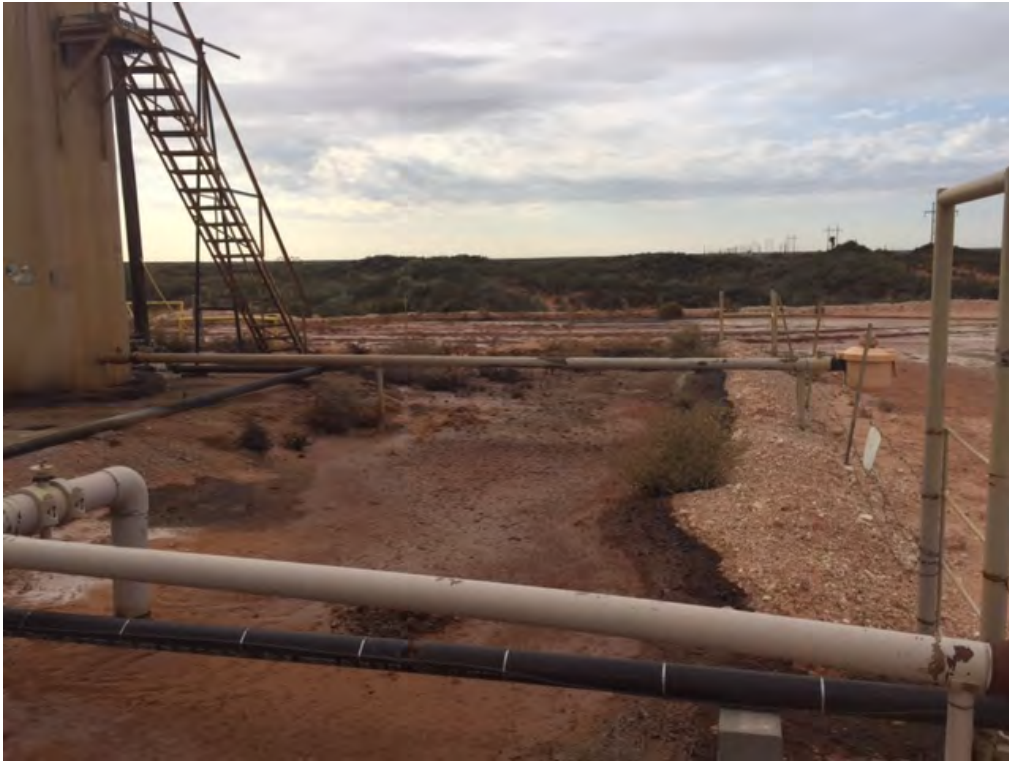
Lost Tank 33 Federal #2 SWD – Release (Looking South-Southeast)
