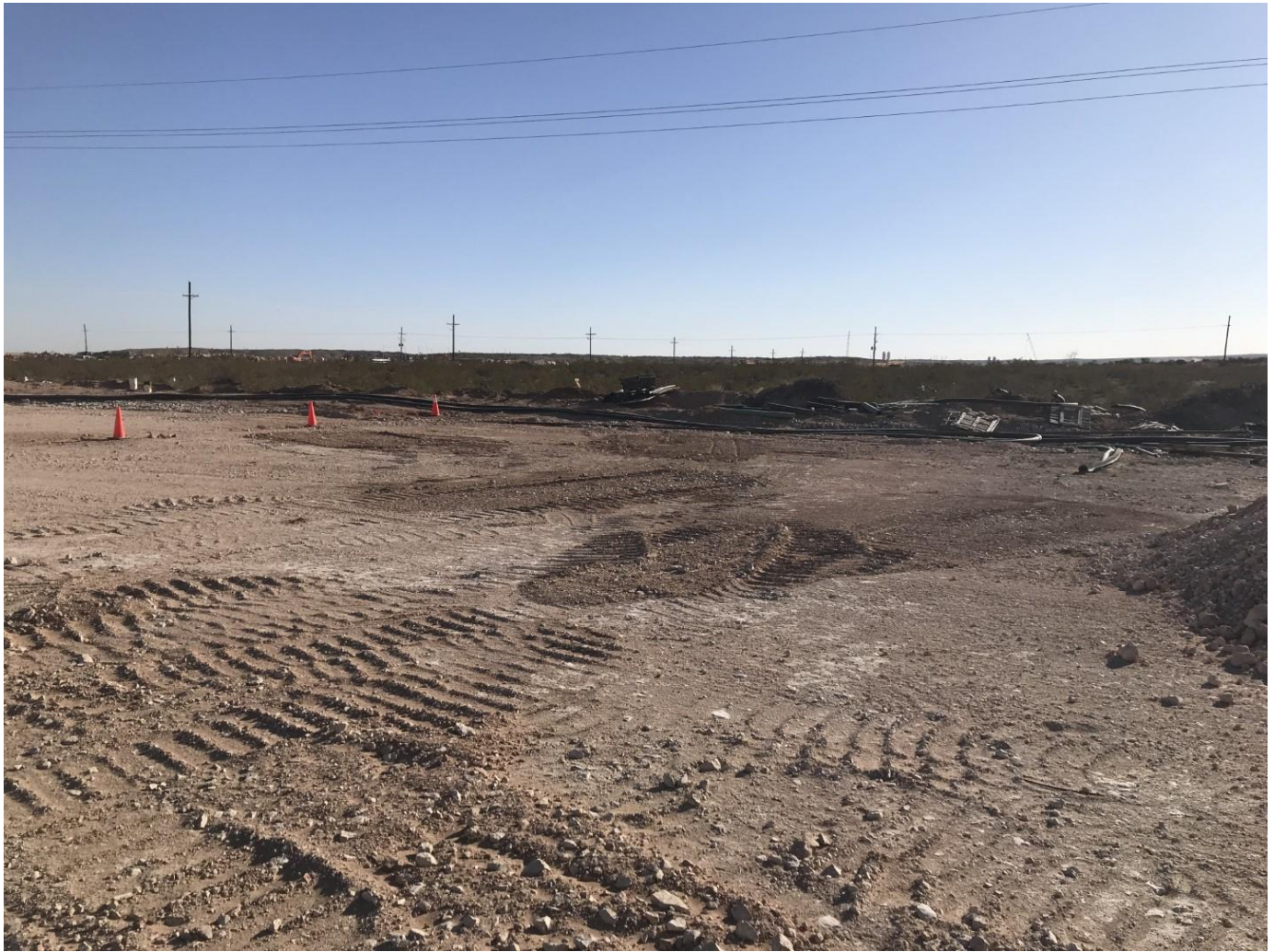
Southeastern view of the contaminated area on the caliche well pad at the commencement of excavation activities.
