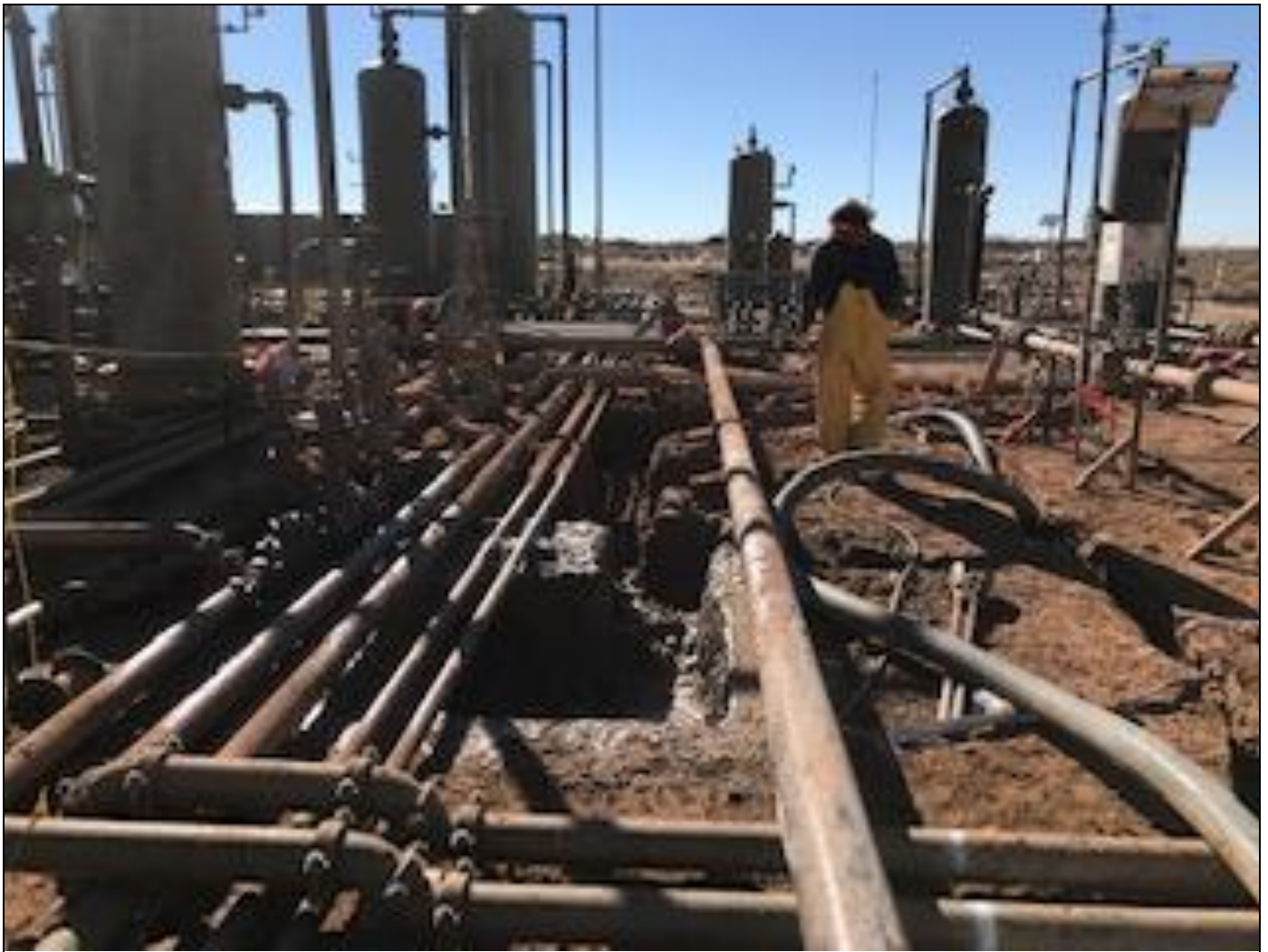
View south of excavation around surface lines within both release areas (2RP-4399 and 2RP-5026)
