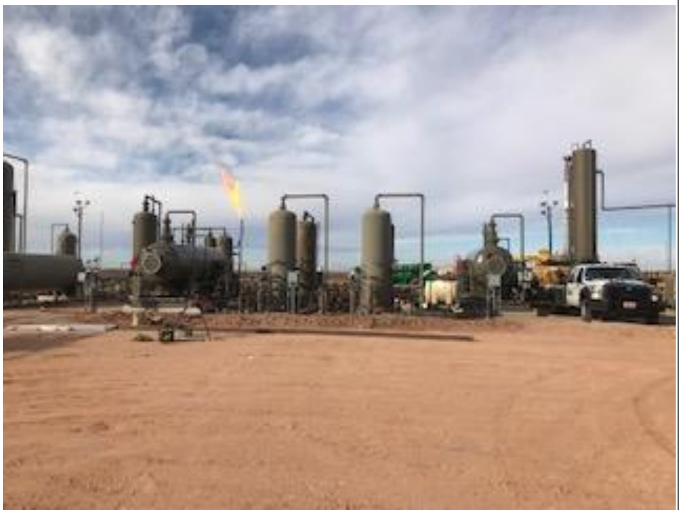
View west of bermed process equipment area
