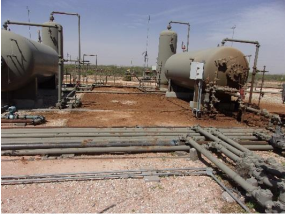
Impacted area inside battery
