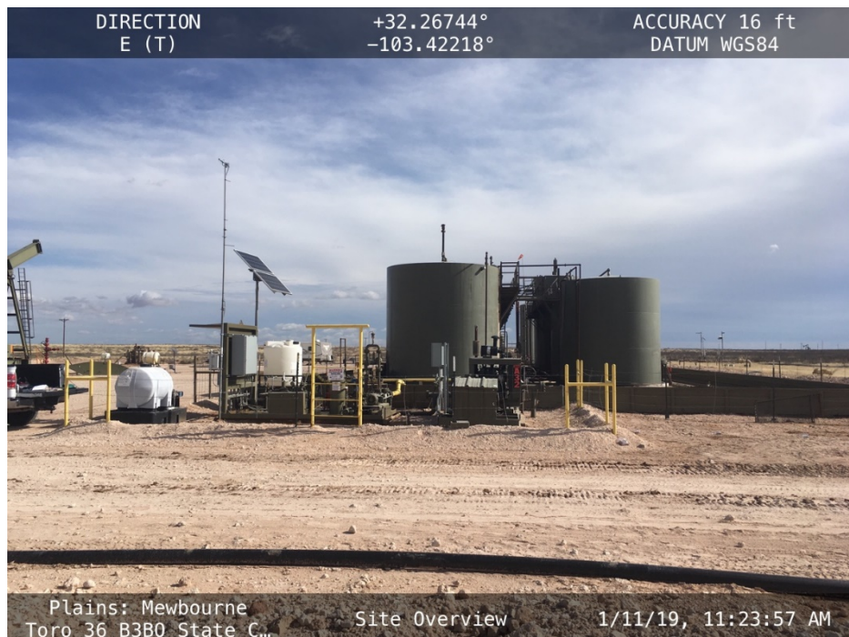
View of affected area after initial response activities facing east
