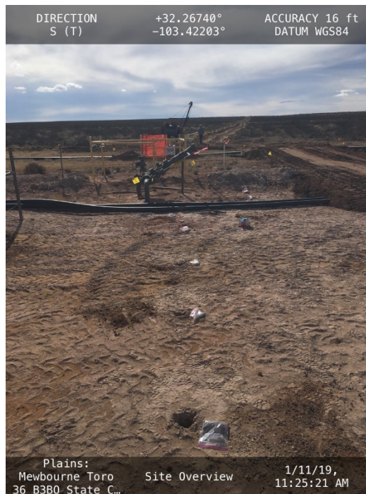
View of affected area after initial response activities facing south
