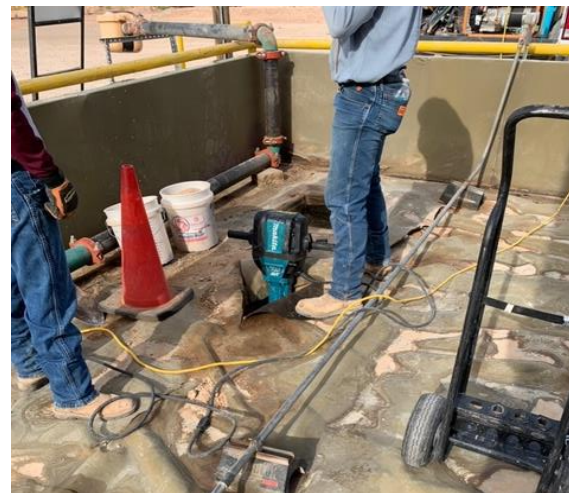
Photograph 3: Utilizing a hammer drill in an effort to advance through formation material within the lined steel berm (BH03).
