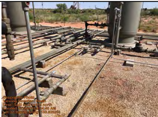
Spill area to the north
