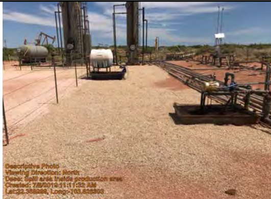
Spill area inside production area
