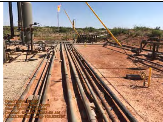
Spill area to east
