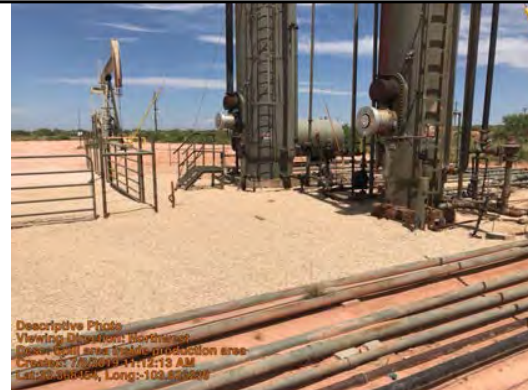
Spill area inside production area
