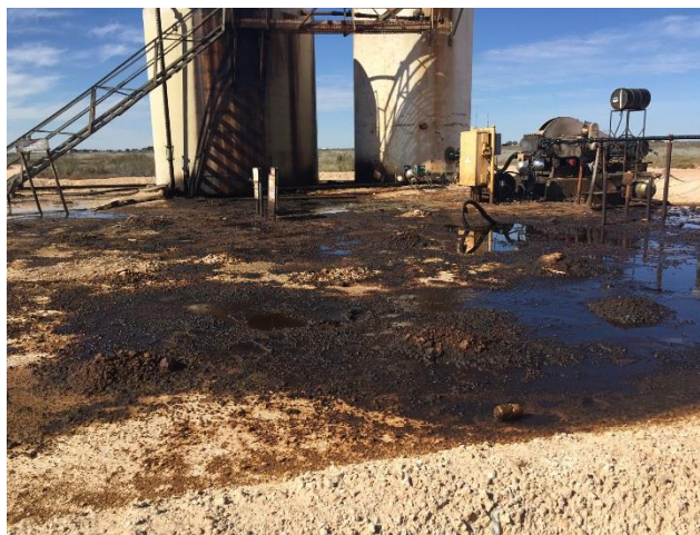
Impacted area facing northwest
