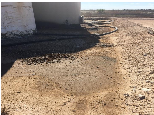
Impacted area west side of tanks
