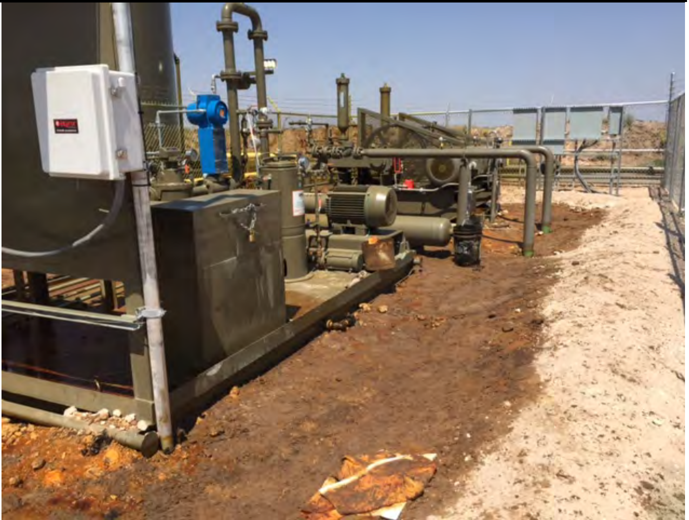
Photo 2: View of surface staining from the initial release, facing northwest.
