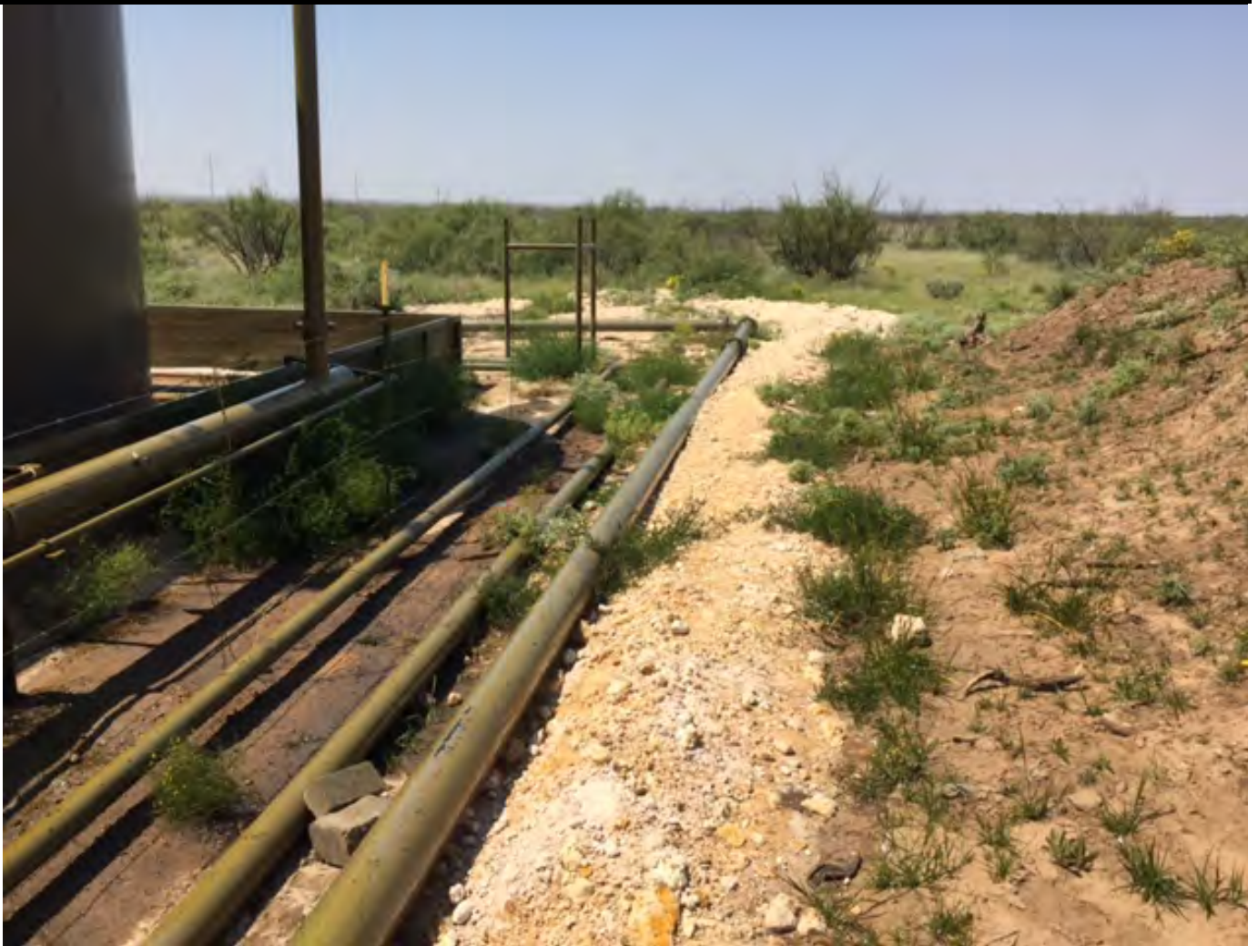
Photo 3: View of surface staining from the initial release, facing west.
