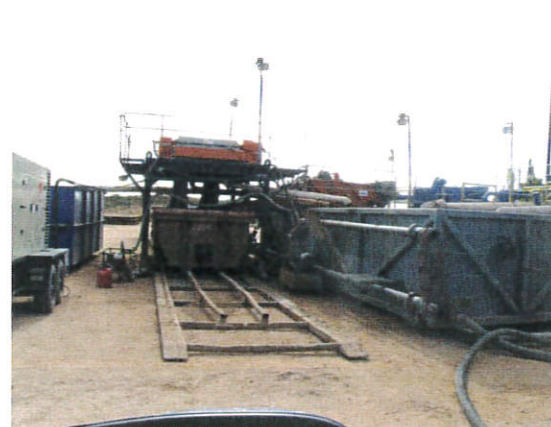
Above: Centrifugal Closed Loop System
